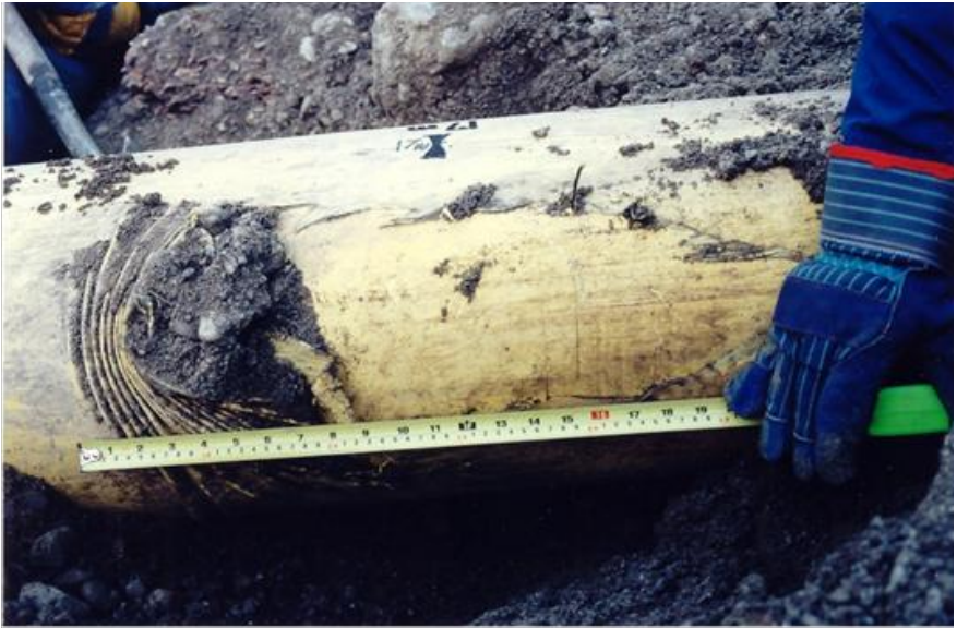
Figure 4.3 Damage to coating on NPS 12 pile from soil movement.
